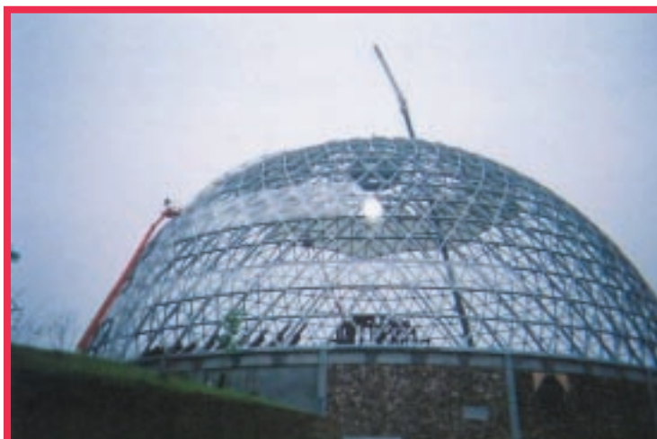
Left: The world's largest glazed geodesic dome takes shape at Omaha's Henry Doorly Zoo.
