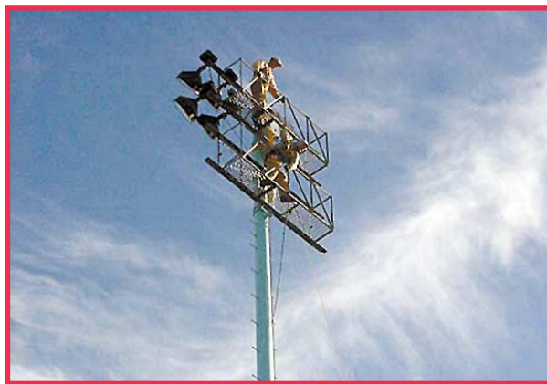
Jay Wells and Brian Ridder work high atop a 90-foot pole to bring a new lighting system to Seacrest Field.
