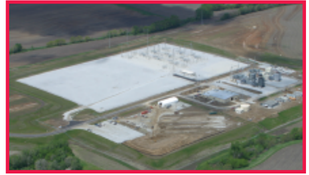
Aerial view of OPPD Cass County combustion turbines
