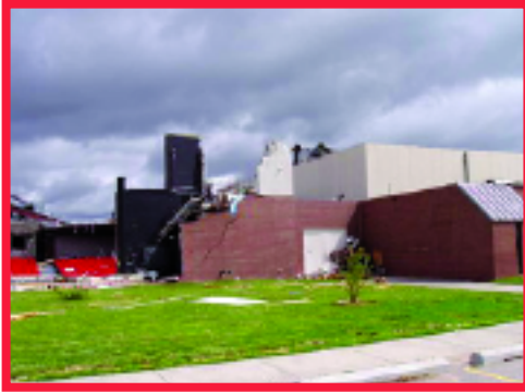
Norris High School Tornado Damage
