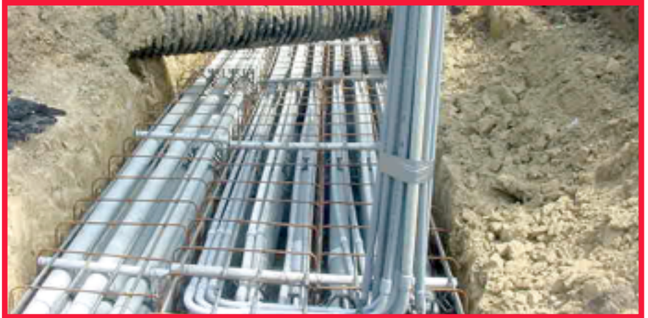
Concrete Encased Duct Bank
