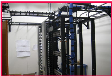
Data Racks Installed
