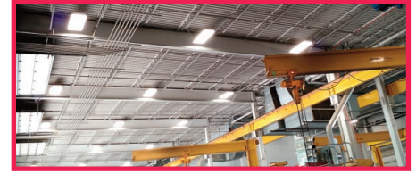
McAninch Maintenance Shop with 8-lamp T5HO fixtures
