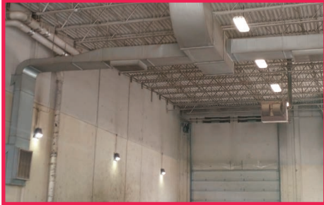
McAninch Wash-Bay with LED wall-packs and T5HO Vapor-Tight fixtures
