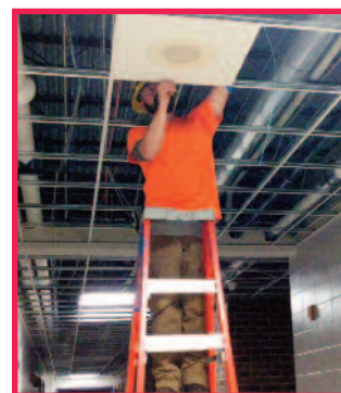
Travis Briggs, Low Voltage Foreman, installing a paging speaker for the Johnston Middle School Remodel project.
