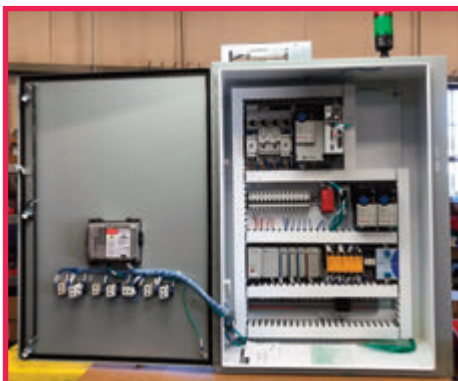
Example of panels being built for Eaton
