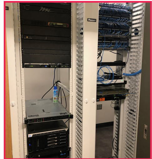
New Corporate IT Server Room
