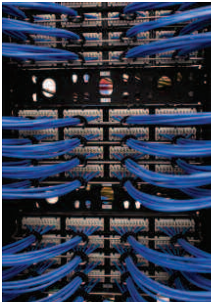
Commonwealth Electric Co. of the Midwest deployed data wiring, technology and overall power services as part of the library's remodel.
