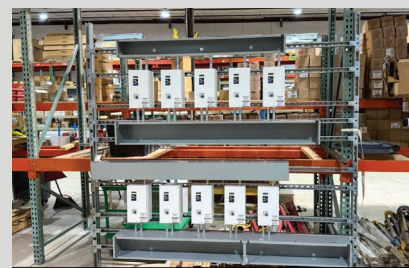
Motor starter racks from Des Moines.
